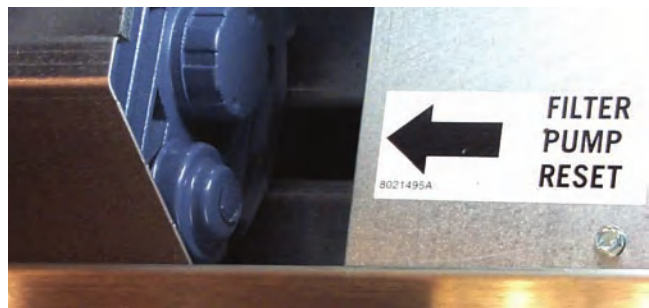
Reset switch location: New-style FPIII
